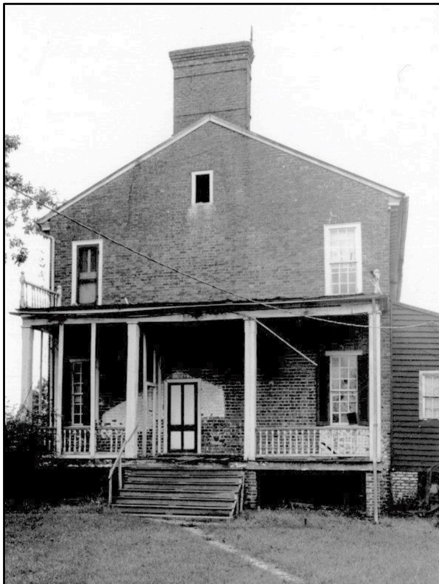
Figure 5: This photo shows the side porch on the east elevation of the main dwelling from the 1972 Survey and NRHP nomination. Note the condition of the porch, the second-floor door on the left of the image, and the porch door on the first-floor level. (Image courtesy of VDHR Archives, Resource ID #134-0027)
