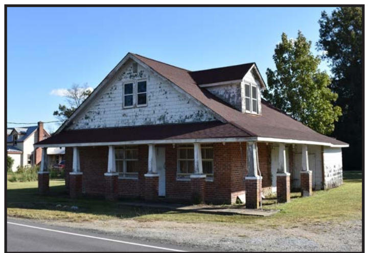
Figure 5.19 - Ginns Store in the southern half of Virginia Beach. This is an example of disrepair that can occur due to vacancy and neglect.
