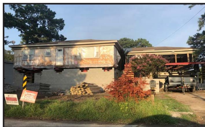
Figure 5.16 - Elevating properties has become a common action in flood-prone areas to protect them from water inundation. While this is a FEMA-approved method, it is not an appropriate option in all situations as the source and magnitude of flood risk vary by property. Therefore, best practice is to tailor mitigation to the specific circumstances of the site and buildings.
