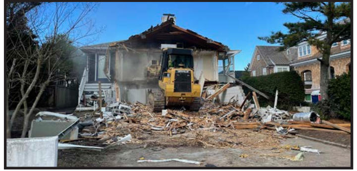
Figure 5.8 - The demolition of historic cottages in the North End is a recent trend as property values often make preservation less attractive to property owners without public policy to balance costs and promote the community benefit.
