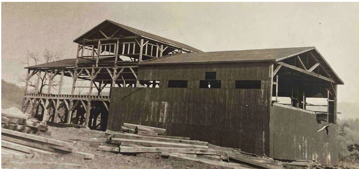
Figure 5 – First mill building under construction in 1920-1921. This two-story building was located immediately south of the existing brick power plant building. Courtesy Bath County Historical Society.
