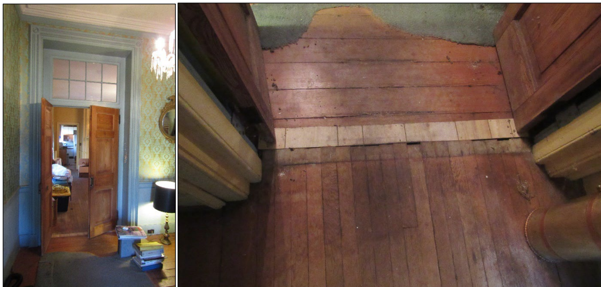
Photo 2: (Left) View of Double-leaf, Paneled Doors (Wagner and McDonald 2020). Photo 3: (Right) Flooring Between Circa-1811 Portion and Circa-1923 Addition (Gordineer 2024).
