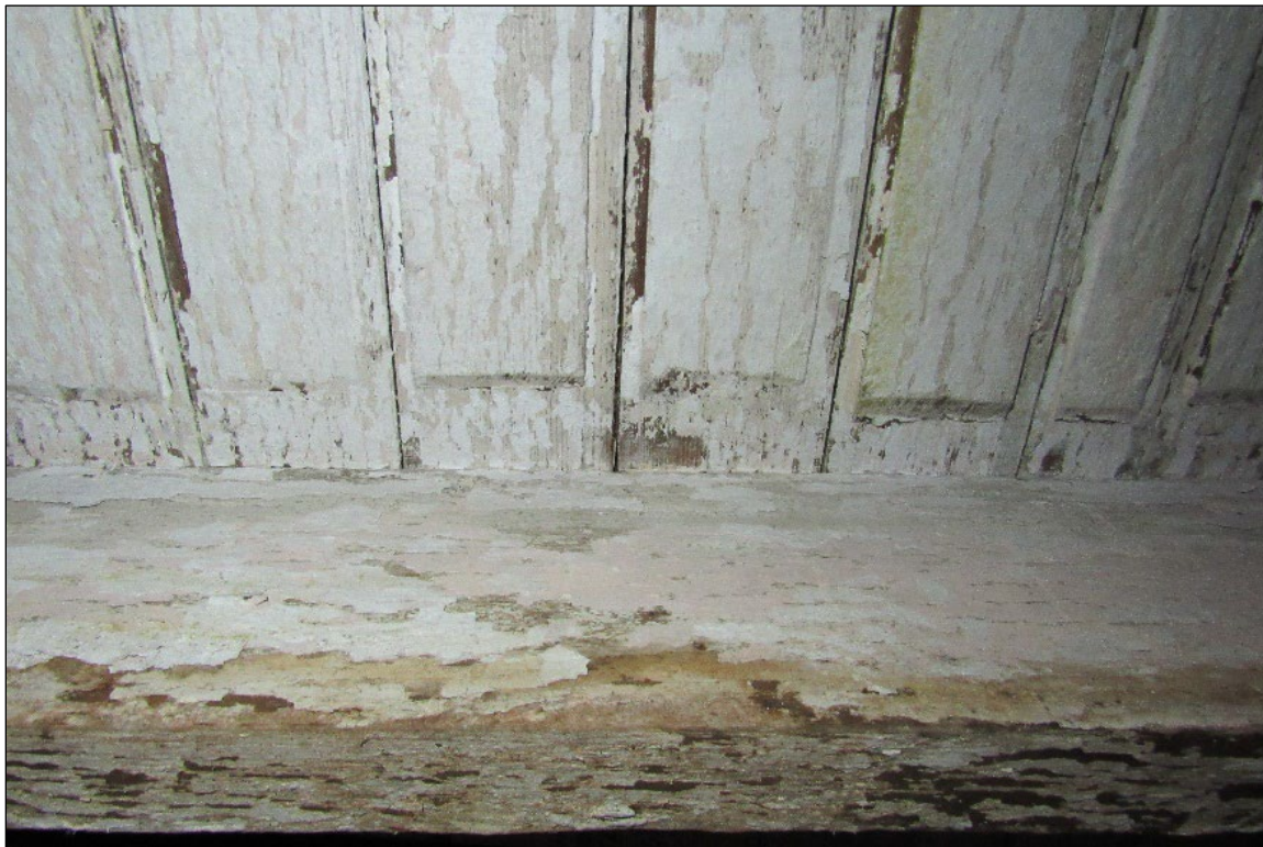
Photo 4: View of the Underside of First Story Flooring from Basement Showing Gauged Floorboards (Gordineer 2024).
