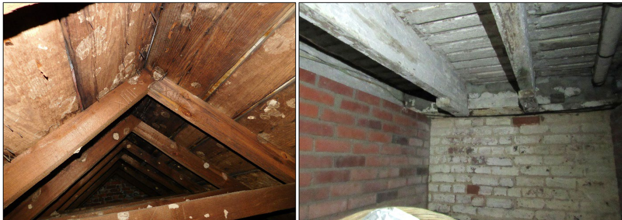
Photo 8: (Left) View of Numbered Supports within Attic of Core (Wagner and McDonald 2020). Photo 9: (Right) View of Flooring Joists in Basement of Core (Gordineer 2024).
