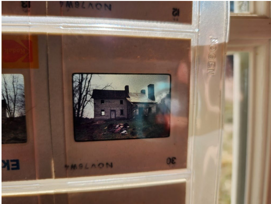
Figure 2. A Kodak negative of the back northern portion of the house, taken by William Miner, shows the property's condition at the time of purchase. Note the windows and condition of the roof. 11
