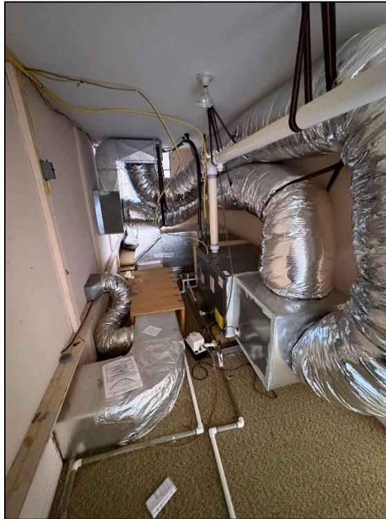
Figure 10. HVAC equipment in the second story.
